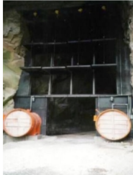
Rear Portal, Ventilation Equipment
